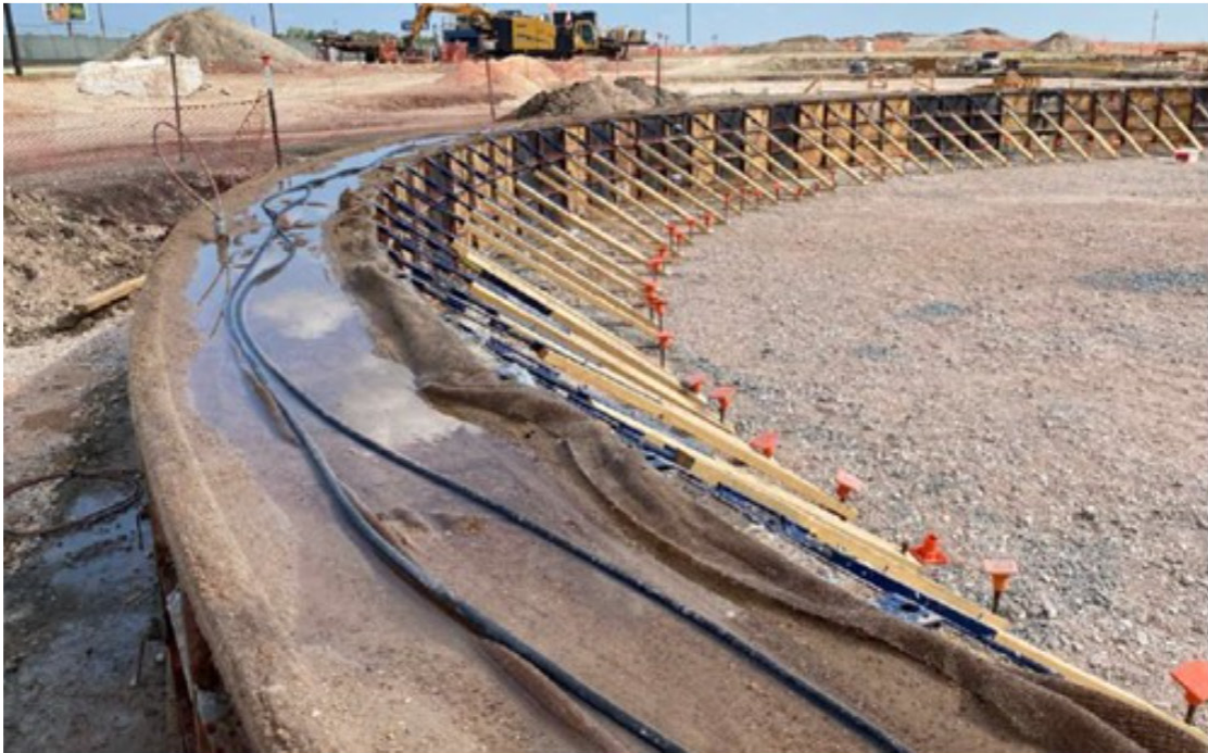
Concrete foundation for one of the tanks dries through a wet curing process.
