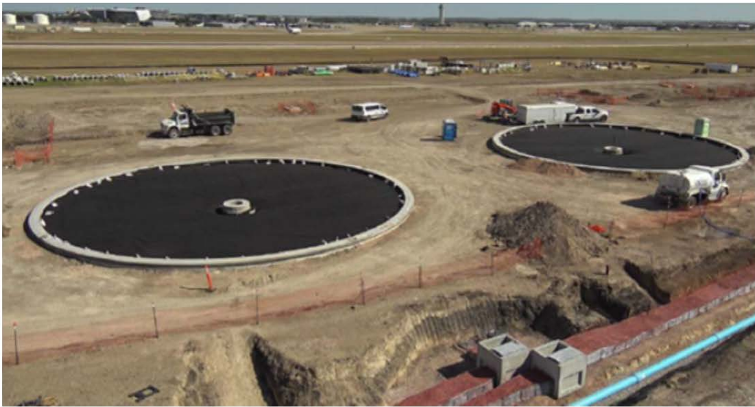
Tank liners placed inside concrete rings that are 3 feet tall and 2 feet thick on top of a 5 foot deep compacted soil base course.
