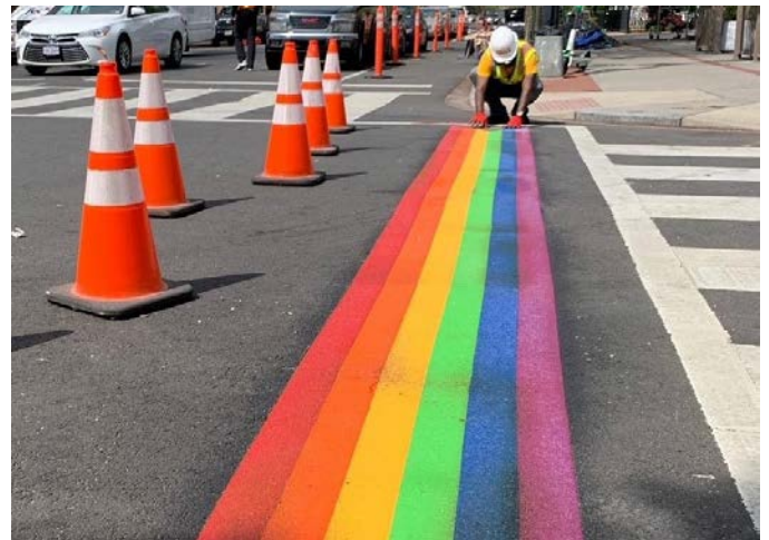
An AROW program installation at a crosswalk on 17th Street.
