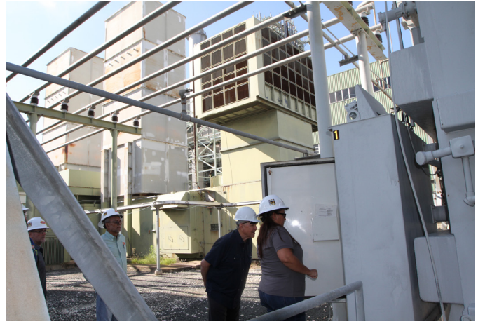
ERCOT inspects Austin Energy peaker units at Decker Creek Power Station.
