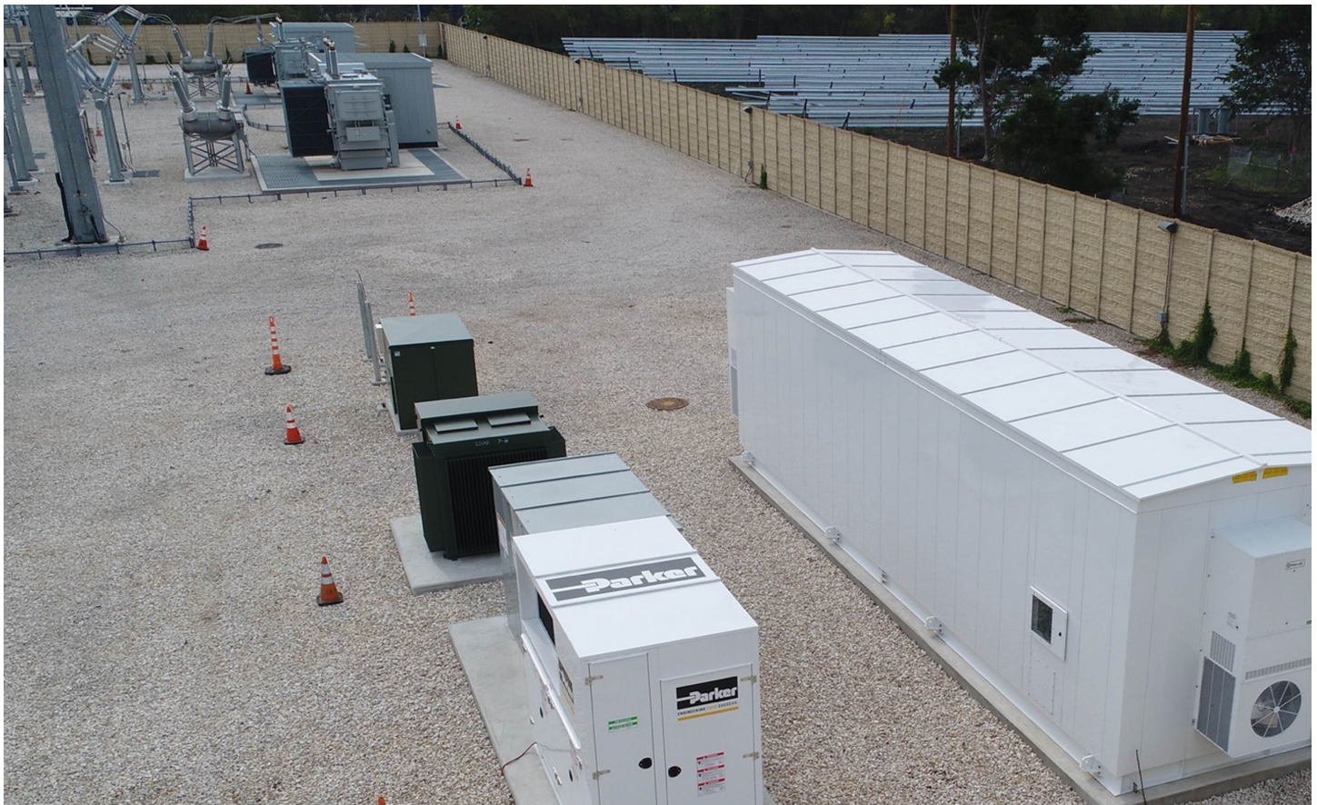
Austin Energy's Kingsbery Energy Storage System is located in a substation and interconnected next to the La Loma Community Solar array.
