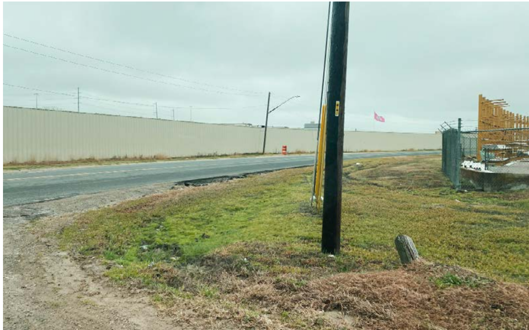
Broken street connections due to US-290
