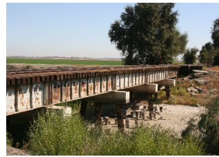
Many significant structures, including railway, bridges, culverts, and crossings are aging and obsolete.
