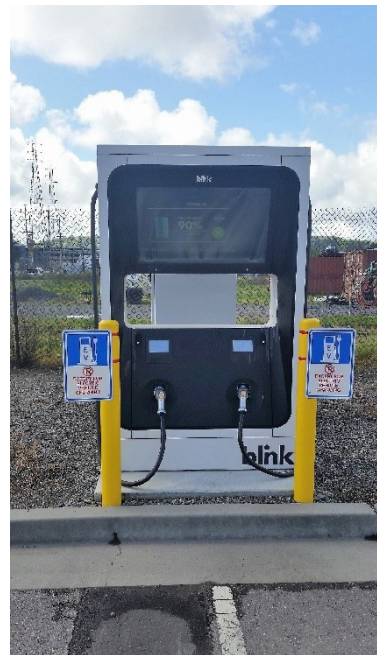
Figure 6-5: Electric vehicle charging station
