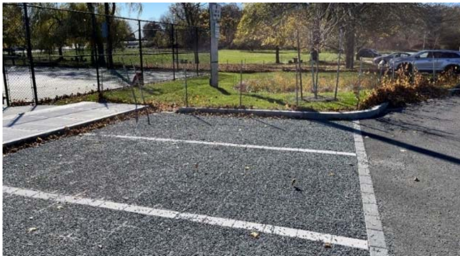
Figure 11. A Reconstructed Parking Lot in Salem, Massachusetts, designed with Permeable Pavers. Image Source: AECOM.
