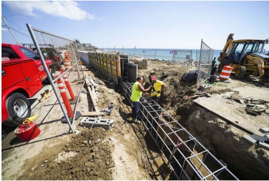
Figure 19. The Matunuck Beach Road Seawall under construction. Image Source: The Boston Globe .
