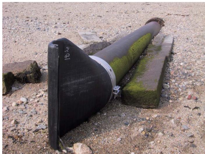
Figure 13. Example of a Duckbill Backflow Prevention Device at Juniper Beach in Salem, Massachusetts. Image Source: Barbara Warren, Salem Sound Coastwatch.
