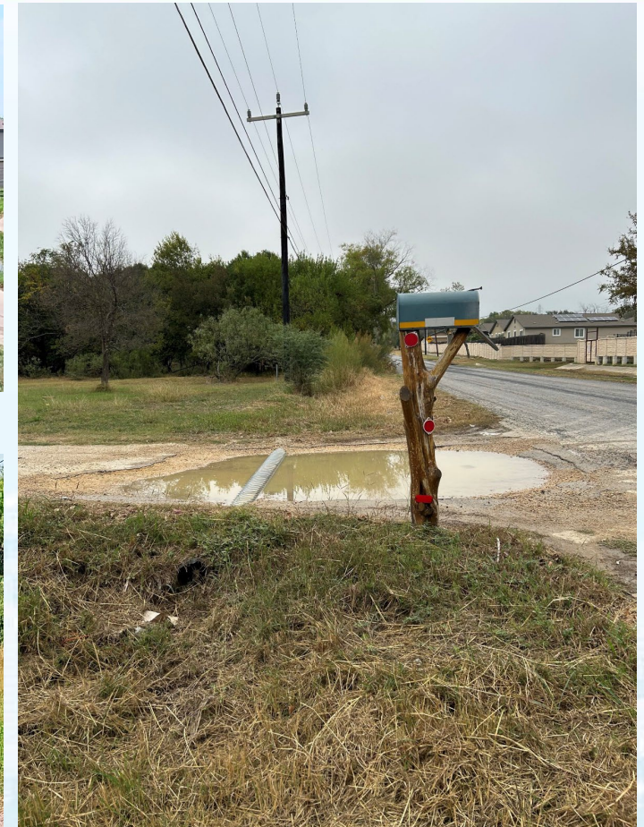
Ponding at a driveway on Southwell
