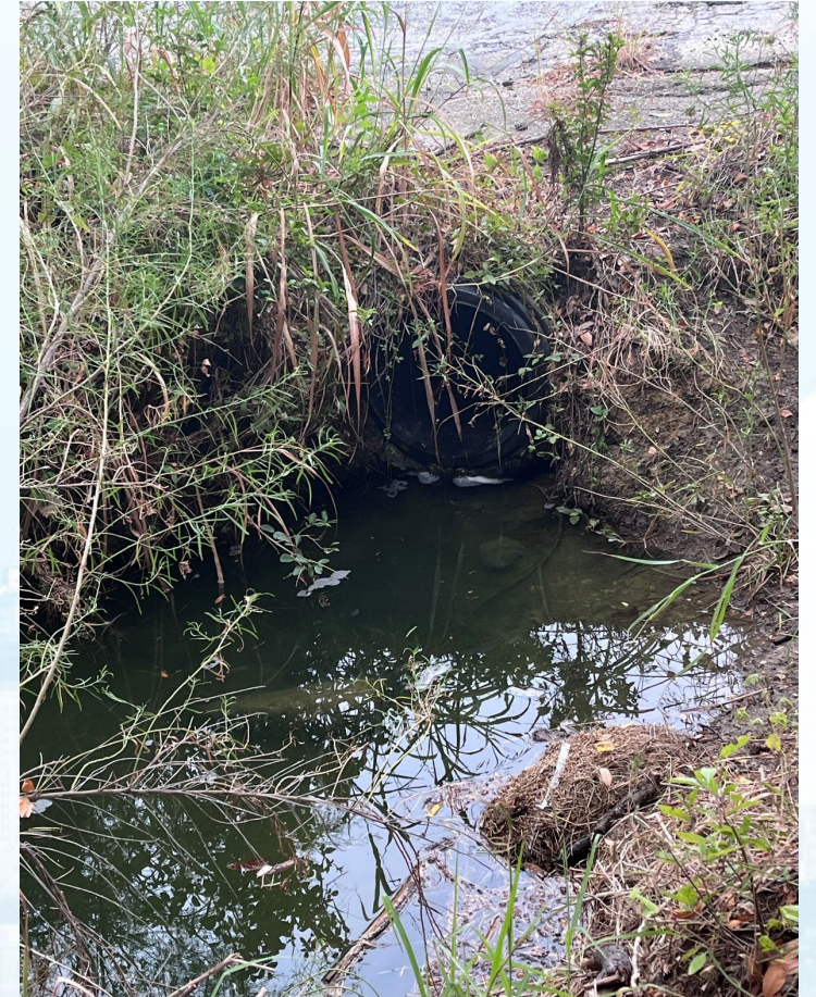
Culvert overgrown with weeds – Facing East
