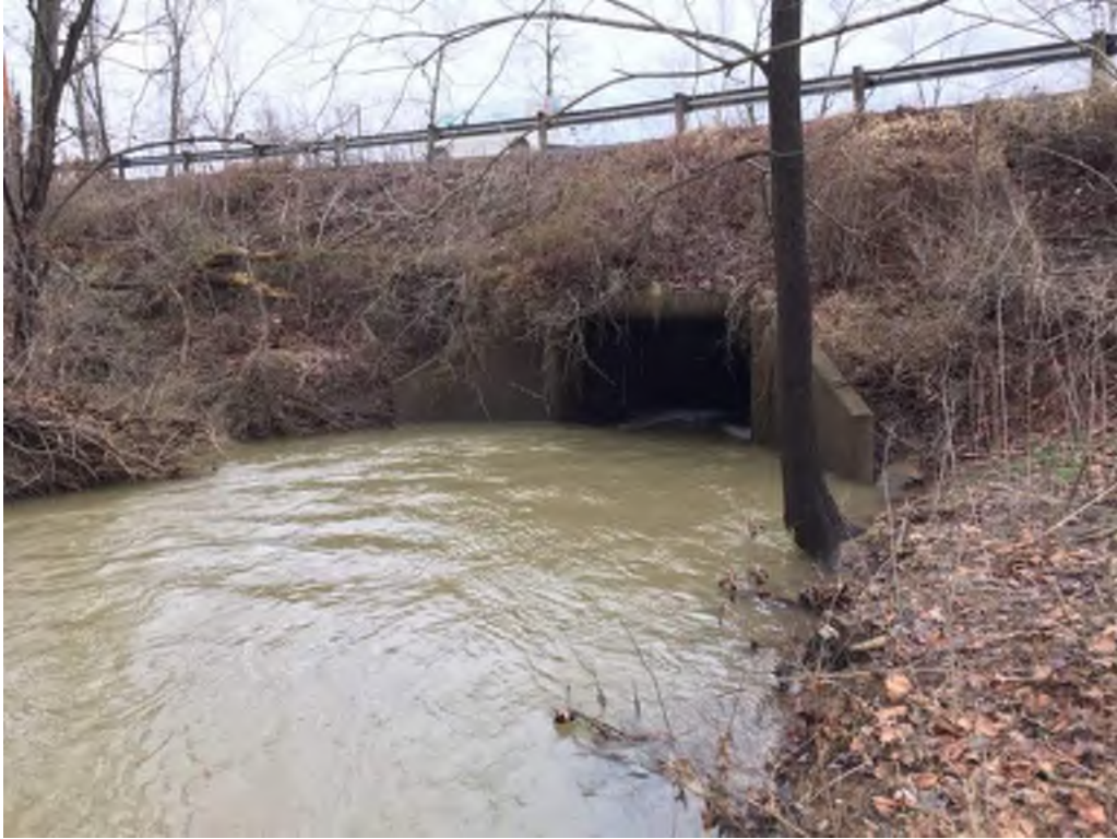
Photograph 39. MG-2661 / Cobun Creek Culvert, Morgantown, Monongalia County From flood plain south of Greenbag Road, facing north
