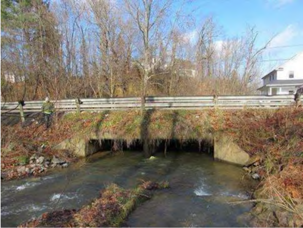
Photograph 41. MG-2666 / Aaron Creek Box Culvert, Morgantown, Monongalia County South elevation of structure, facing northeast (WVDOH 2018)
