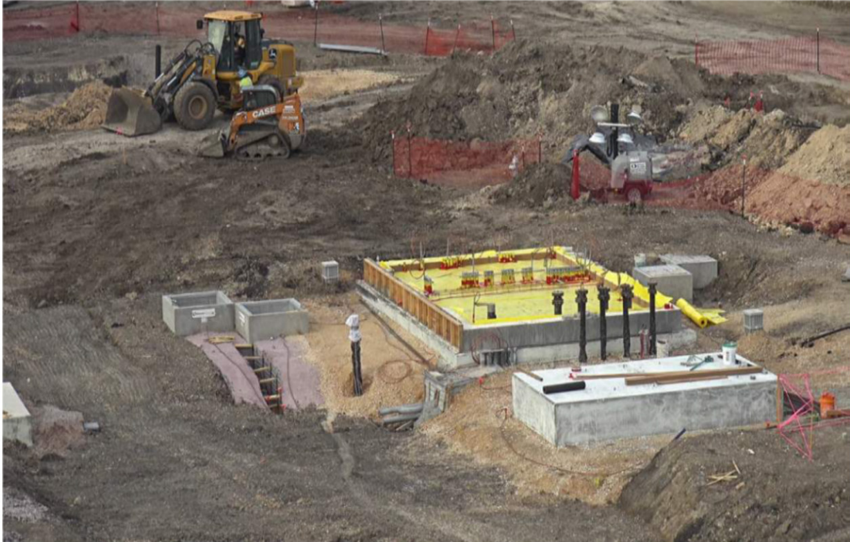
Fire Foam Building and generator pads
