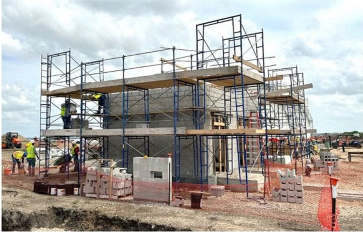
Fire foam pump house
